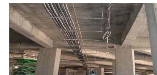
MC cable using trapeze support system
