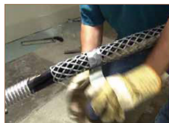
Securing basket grip to conductor assembly to avoid pulling conductors out of armor
