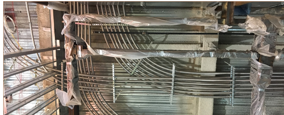
Wire Mesh Support System with Type MC cable
