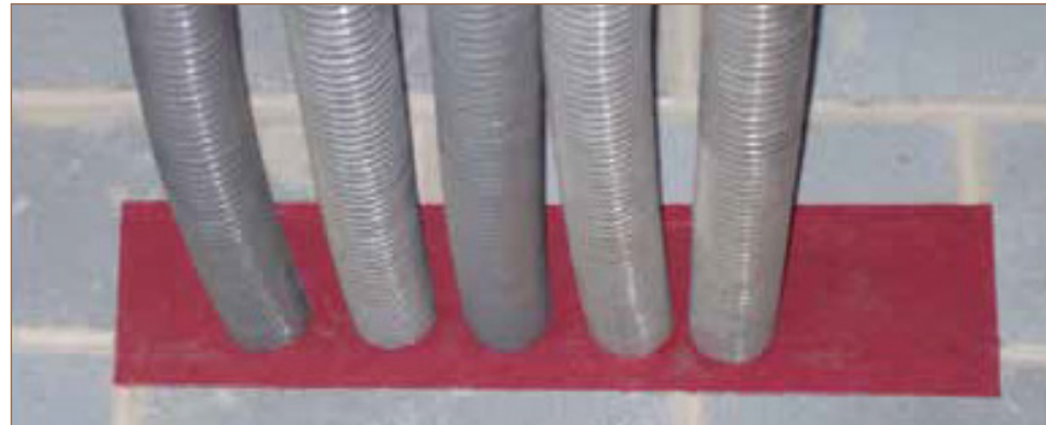
MC feeder cable in wall with fire stop
