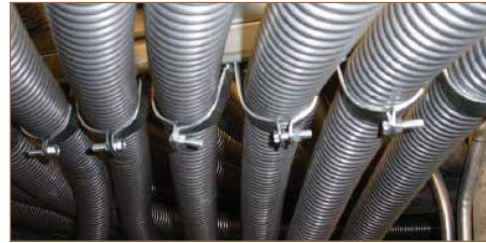
MC cable secured every 6' with straps and clamp
