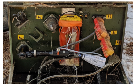
Figure 2: MIC Injection in a low-profile transformer
