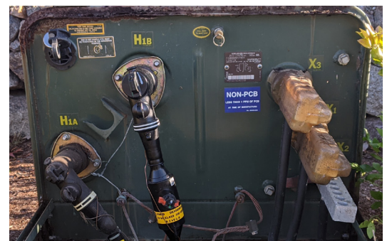
Figure 2: MIC termination in a transformer.
